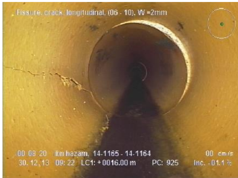
Figure 54, CCTV Image with Cracks and Displaced Joint
