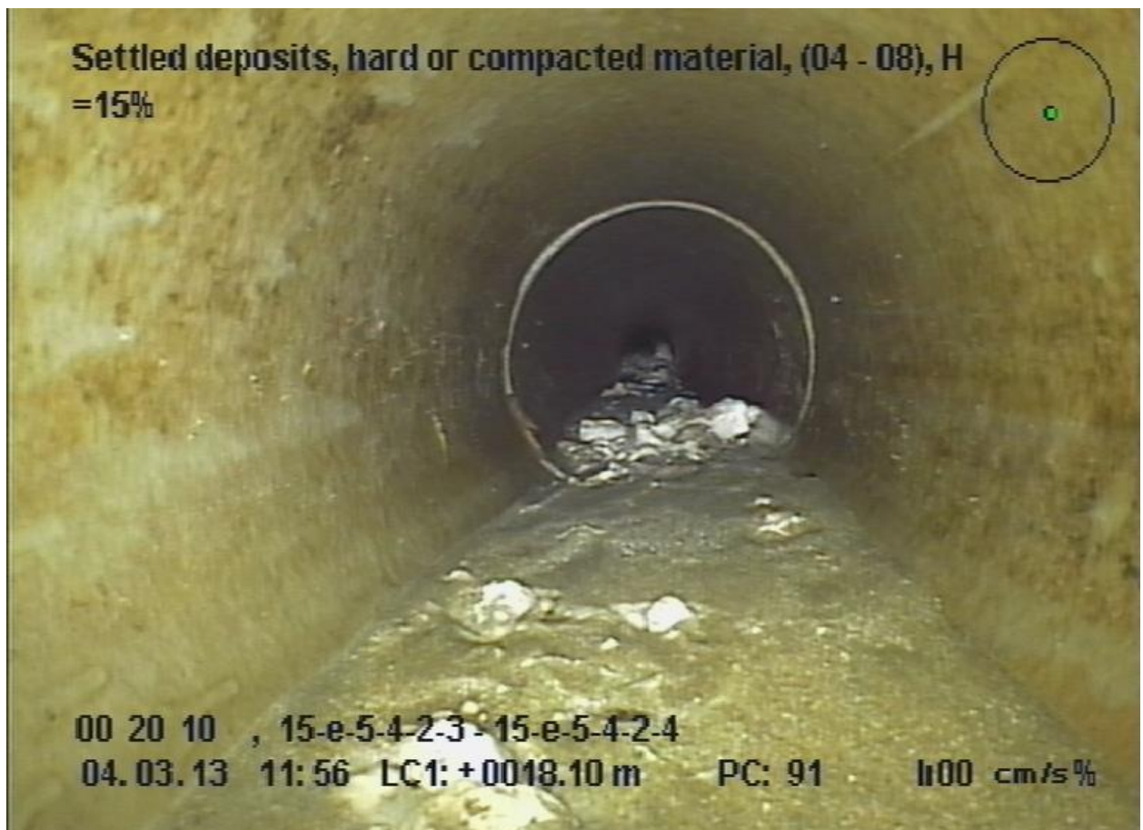
Figure 15, Example of settled deposits from a CCTV Camera Footage
