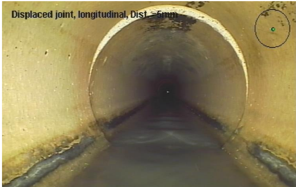
Figure 17, Example of a displaced joint from a CCTV Camera Footage
