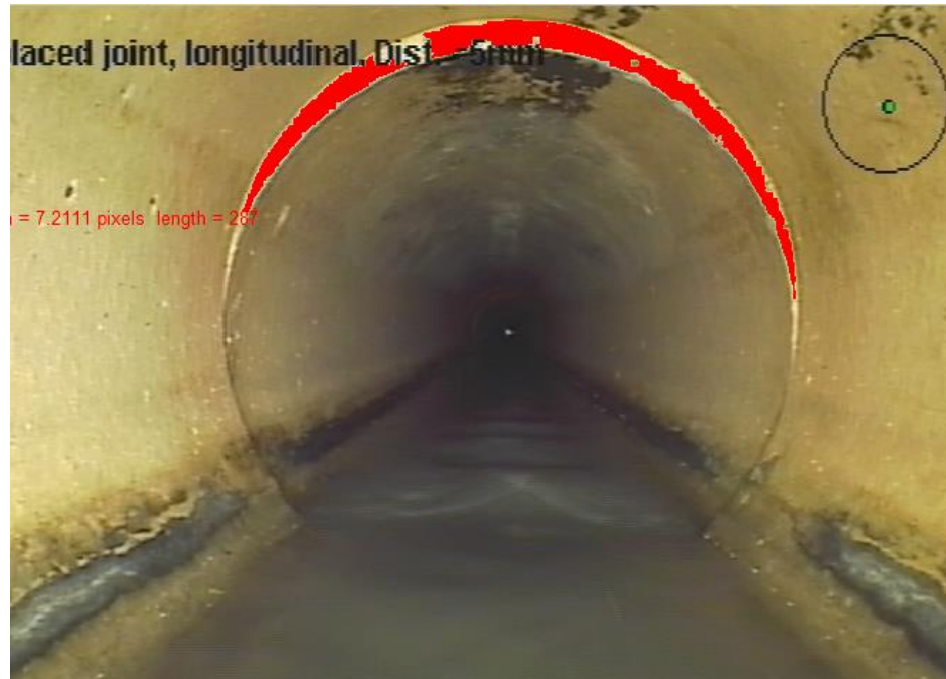
Figure 61, Example of Detection of Displaced Joint
