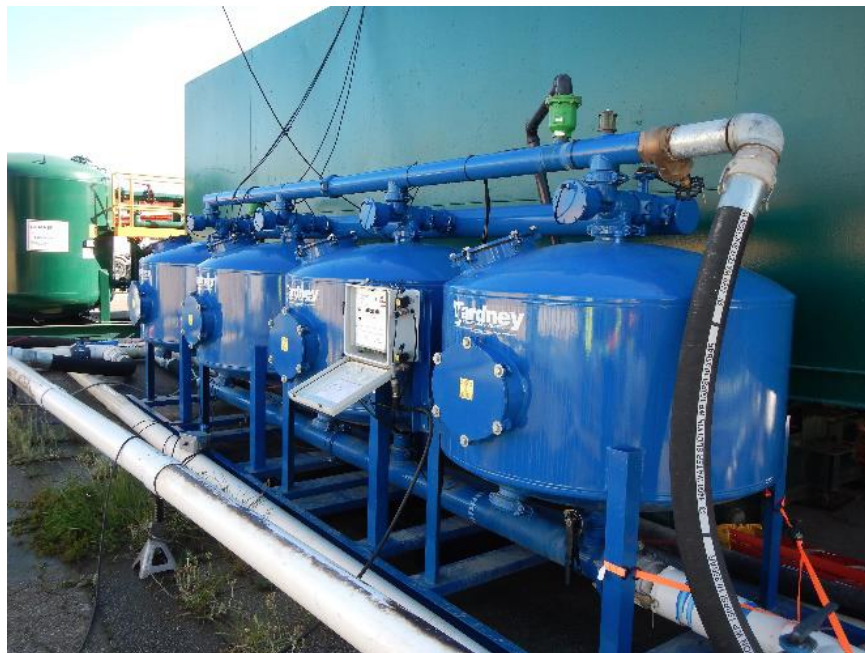
Figure 11: Multimedia sand filter [38]
