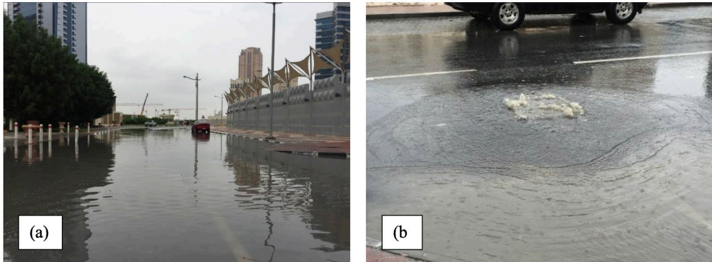
Figure 1: Flooding in Doha, (a) Trapped rainfall-runoff collecting on the low point of a main road in Doha; (b) Example of road drainage network exhibiting capacity exceedance/overflow.
