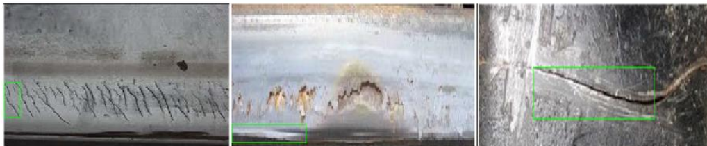
Figure 2. Examples of surface defects [4].
