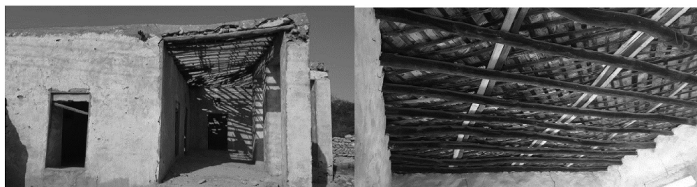
Figure 8. Illustrates the deterioration of buildings in Tinbak as one of its internal weaknesses. On the other hand, its strength appears in the old building that reflects traditional Qatari architecture and traditional roof construction techniques.
