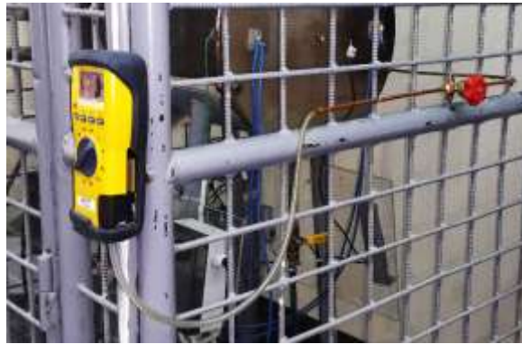
Figure 33 - Lambda sensor piping and connection
