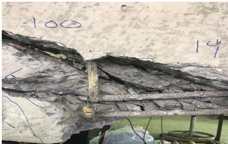
Figure 35. Rupture of the stirrups B-4.
