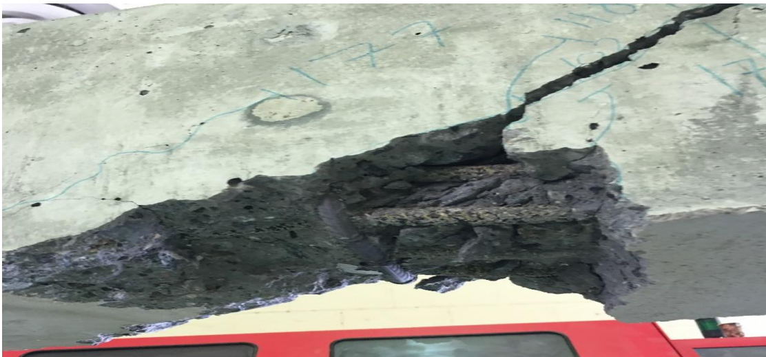
Figure 44. Steel stirrups after failure.
