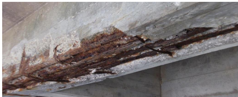
Figure 1. Examples of deterioration.
