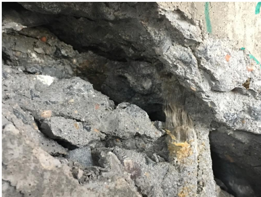
Figure 30. Rupture of the BFRP stirrups.
