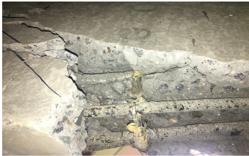
Figure 32. Rupture of the stirrups B-2.
