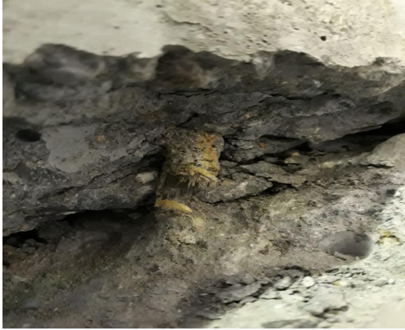
Figure 41. Rupture of the stirrups B-8.
