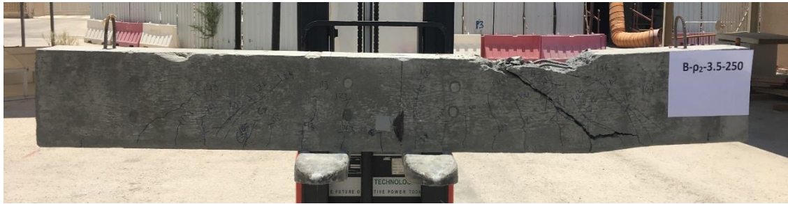
Figure 36. Beam B-5 Shear Compression failure.
