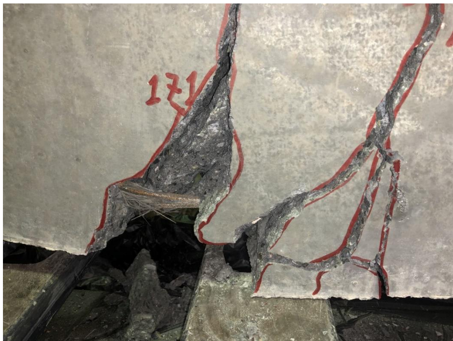
Figure 79: Typical rupture of FRP bars
