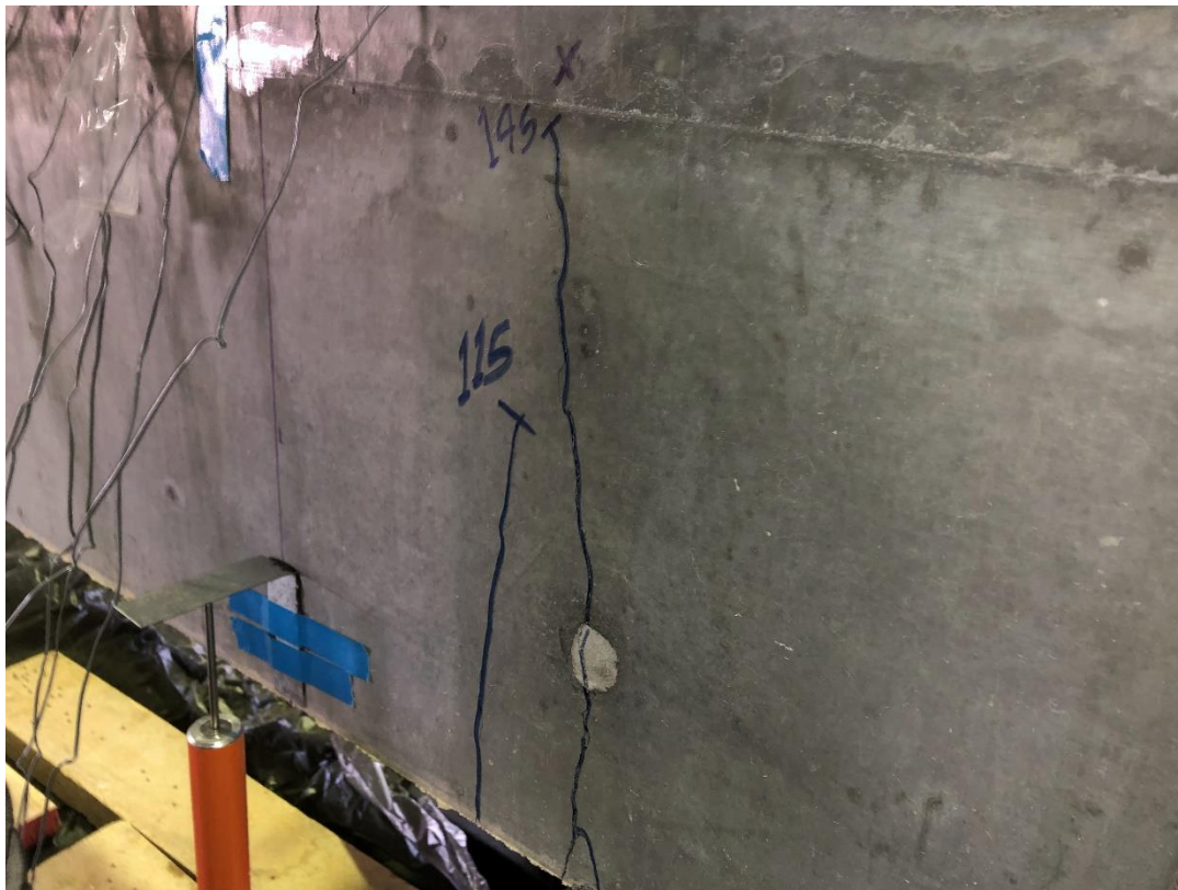
Figure 68: Two cracks of beam 10 (HWBFRP-10-400)
