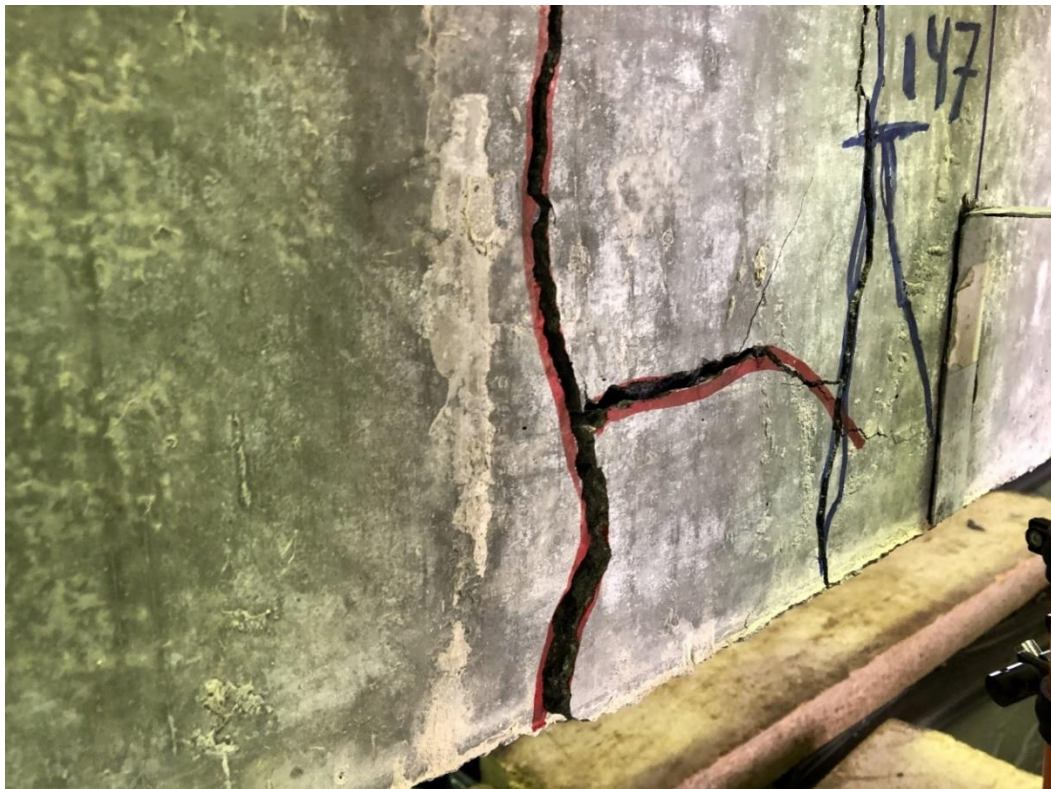
Figure 75: Splitting failure of concrete in the tension zone
