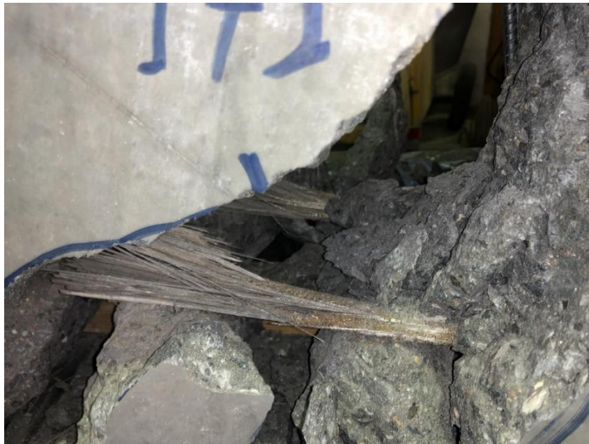
Figure 78: Typical rupture of FRP bars
