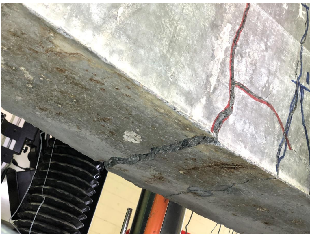
Figure 76: Splitting failure of concrete in the tension zone
