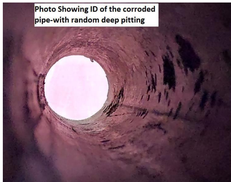
Figure 4. Showing ID of failed spool
