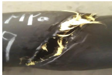
Figure 5. failed aramid fiber reinforced pipe under internal pressure at 90 °C[31].
