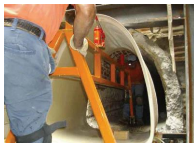
Figure 32. The original concrete pipe while placing the FRP liner since much of its protective liner was missing [116].
