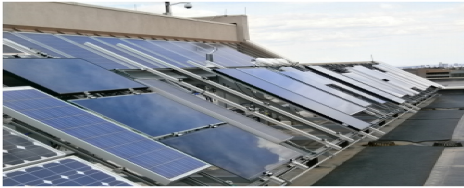
Fig. 4 PV modules deployed at the National Renewable Energy Laboratory [16].
